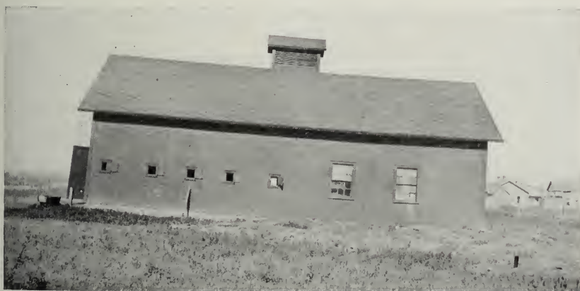
FIG. 47.—Barn of mining company lowered 4 feet at one end. It has been partially restored.
